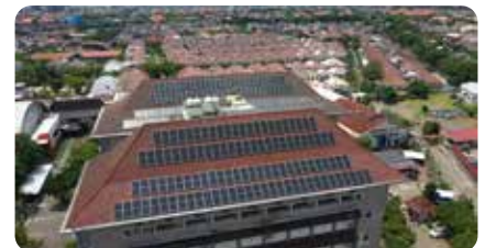
PV Rooftop Kantor Pusat PV Rooftop of Head Office
